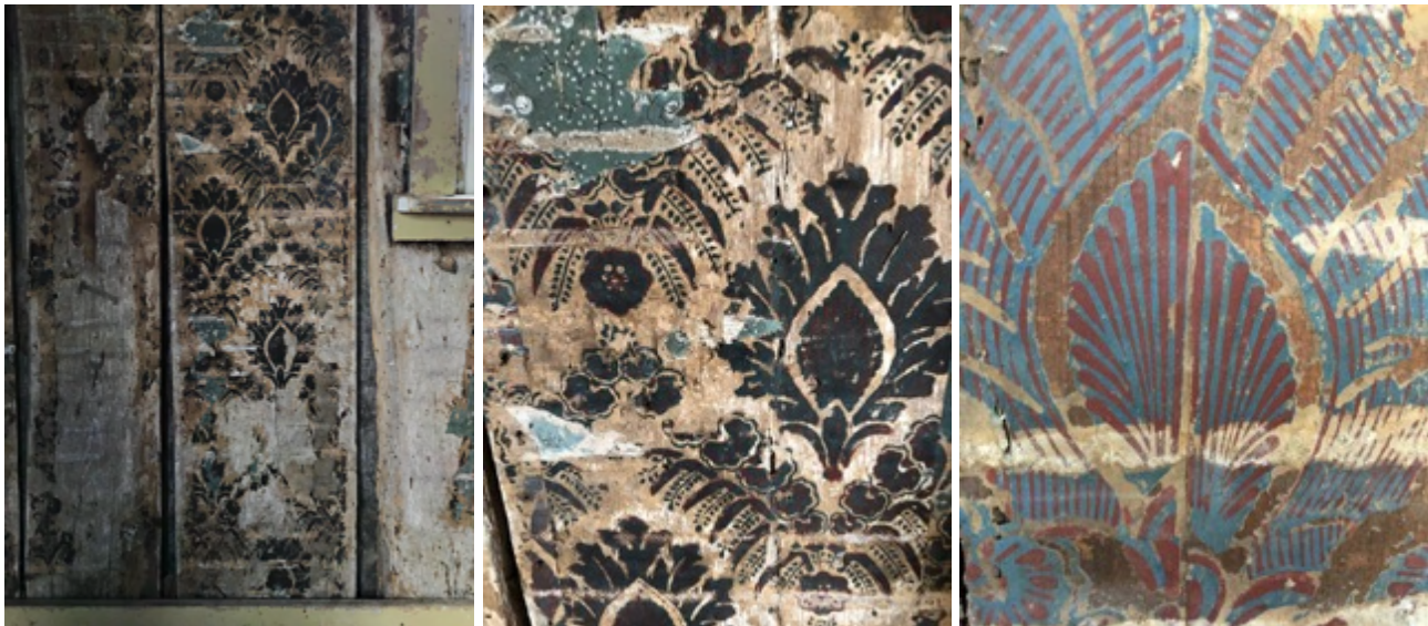
Central plank exhibits offset palmette pattern (left), Detail of palmette with laurel & cascading leaves (center), Wallpaper seam at the center of the palmette installed slightly out of alignment (right)
