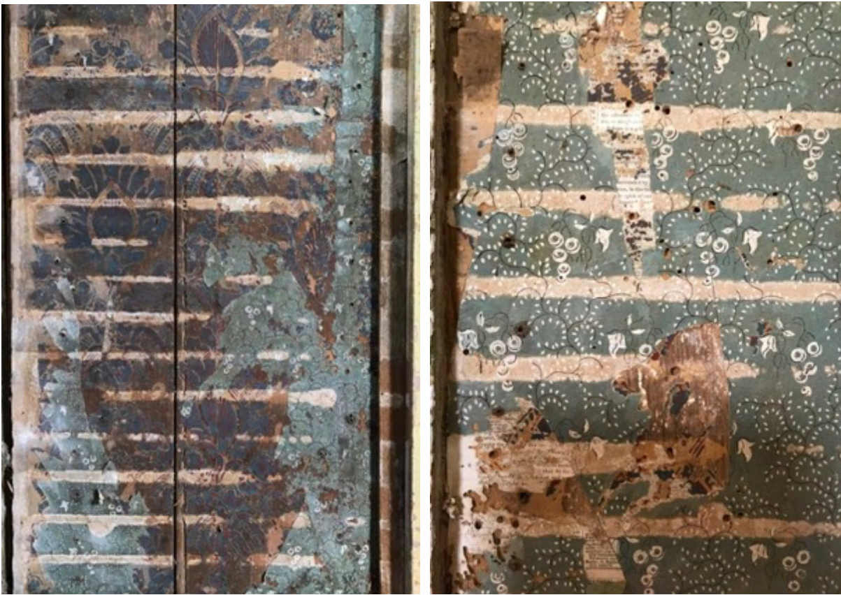
Wallpaper fragments revealed on the original wall surface upon removal of the plaster & lath surface wall.
