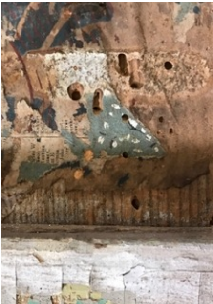
Wood boring insect damage
