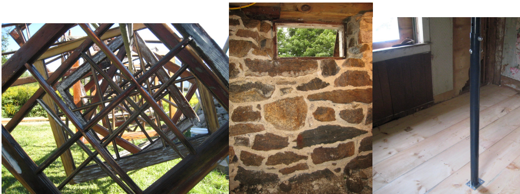
Second phase of restoration included windows, foundations, new pine flooring, endless stabilization, temporary steel posts like this one, and much more. Photos by Diane Gilbert, September 2009.
